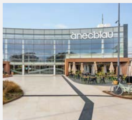
Ànec Blau: completing the façade and adding a new outdoor food court area.
